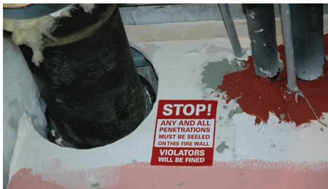
Smoke and fire barrier penetrations are a top cause of Joint Commission citations in hospitals.
